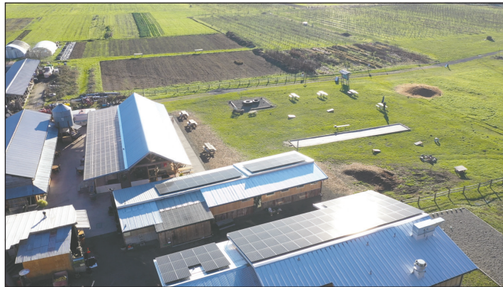
Power Trip Energy Corp has been installing solar arrays for residential and commercial projects since 2003, including this array at Finnriver Farm & Cidery in Chimacum. Courtesy of Power Trip Energy Corp.
