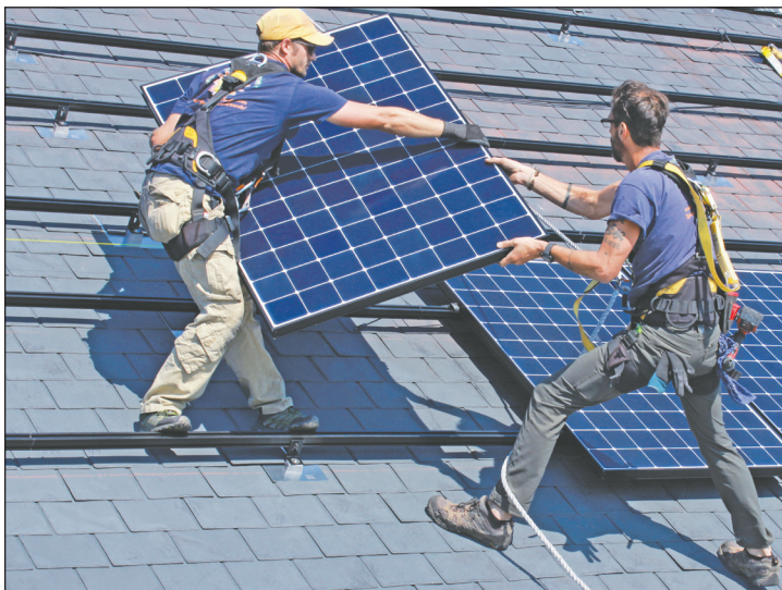
Power Trip Energy Corp are general contractors and electricians, installing approximately two residential solar arrays per week. Courtesy of Power Trip Energy Corp.
